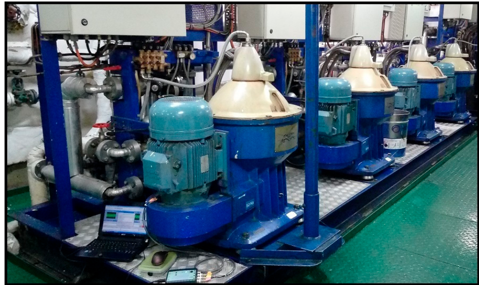
Figure 1. Lube oil centrifugal separator systems.
